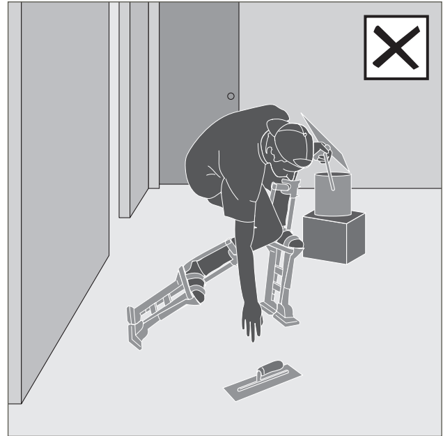
Figure 25 Inappropriate activity whilst on stilts – reaching below foot level stresses the knee, ankle, back and stilts.
